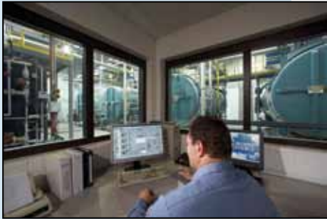
Optimal combustion in a boiler requires adequate air supply in the boiler room.
