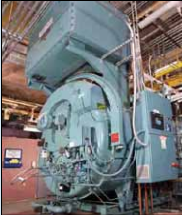
Optimized Boiler Package operating close to 90% fuel-to-steam efficiency.
